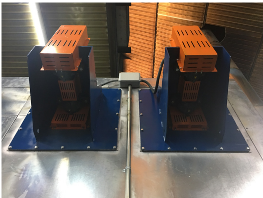
CLIBOS-TR installed in a paint booth oven
